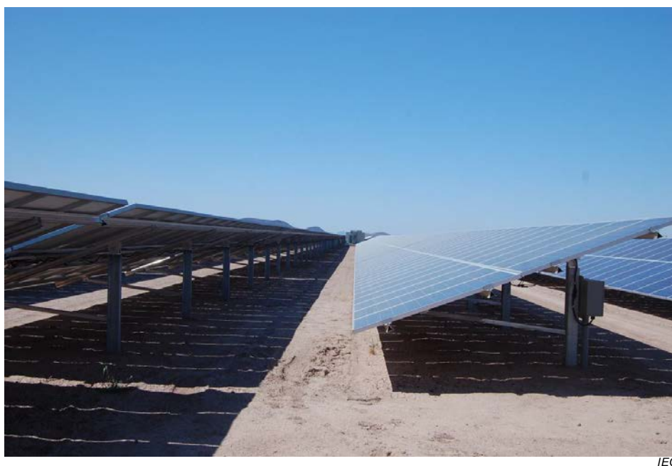
Figure 5 – Example power plant with fixed tilt array
