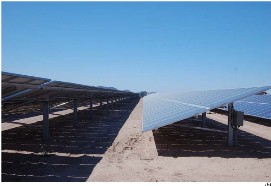
Figure 5 – Example power plant with fixed tilt array
